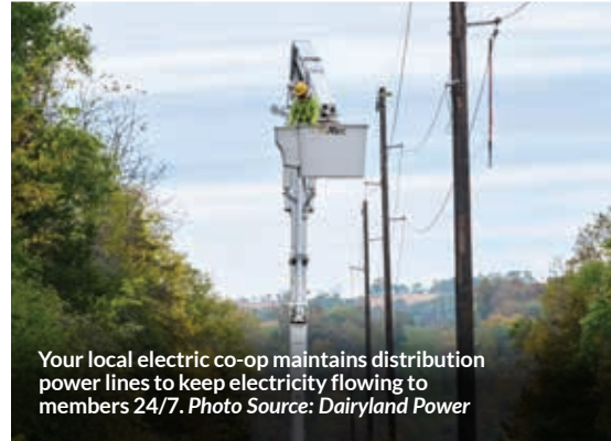
The complex electric grid includes thousands of generators, hundreds of thousands of miles of transmission lines and millions of miles of distribution power lines all working together to keep the lights on day and night. Photo Source: NRECA
